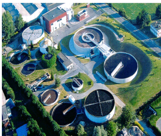
STATION D'EPURATION - HAZEBROUCK
